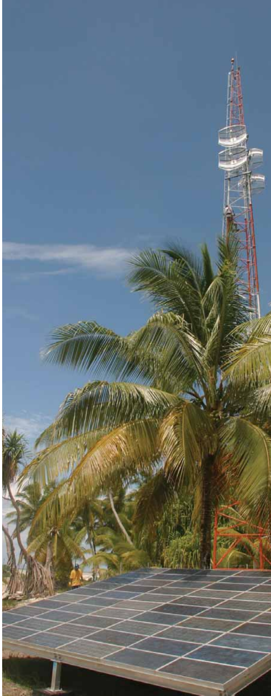
Solar powered microwave station, Kiribati
