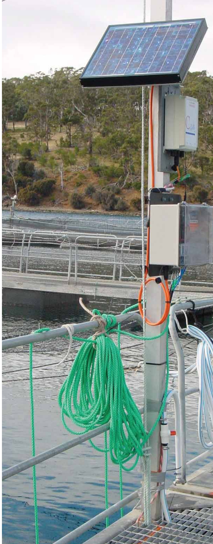
Datacall monitors oxygen and temperature, Tassal salmon farms Tasmania
